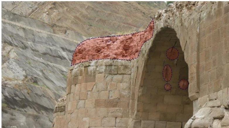
Fig. 8. Damage to the small bridge and moisture dampness under the small arches indicate the presence of decreasing humidity.
