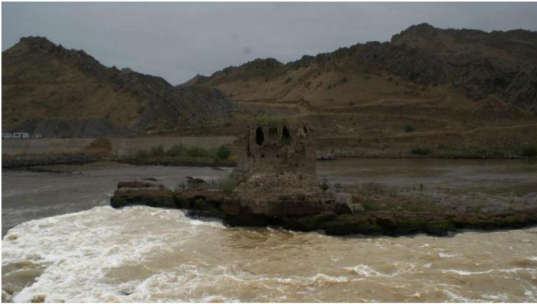
Lack of natural bed in the area of bridge piers
