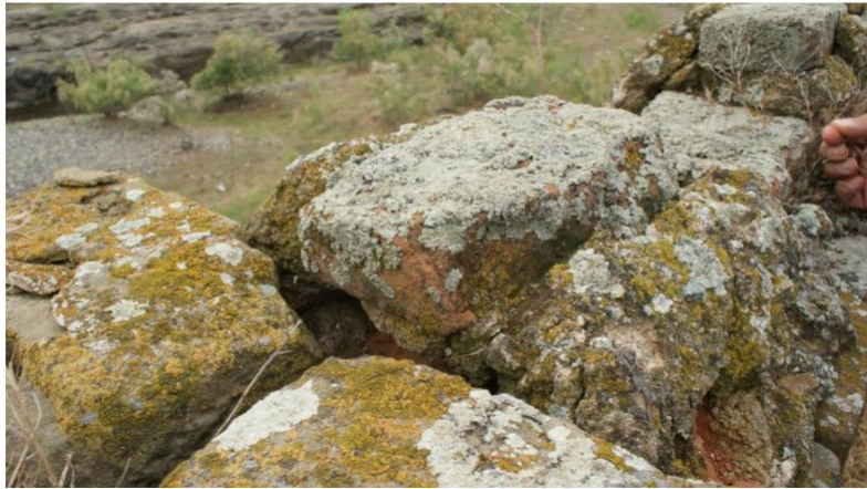
Fig. 9. Growth of microbiologies on large bridge materials
