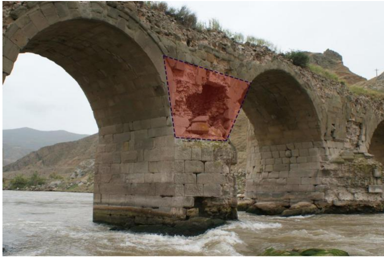
Fig. 7. Destruction of a part of the pier in the small bridge due to the floods
