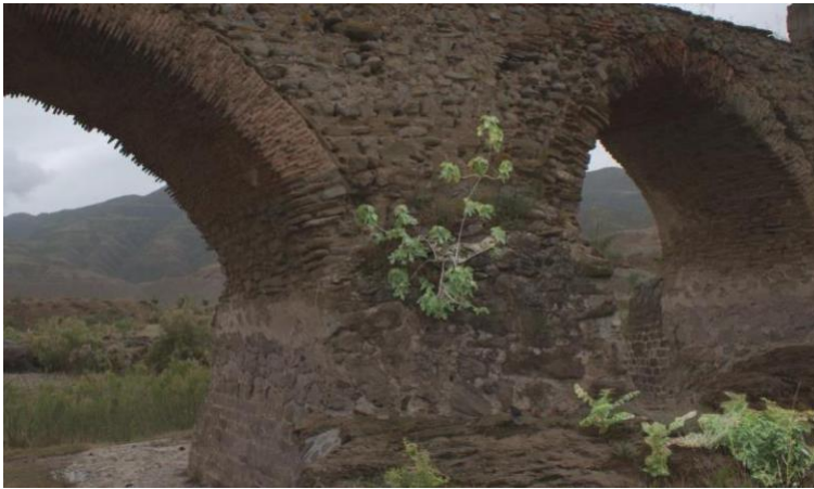
Fig. 9. The growth of shrubs and plants on the piers in large bridge is regarded as a biological damage to the plants.
